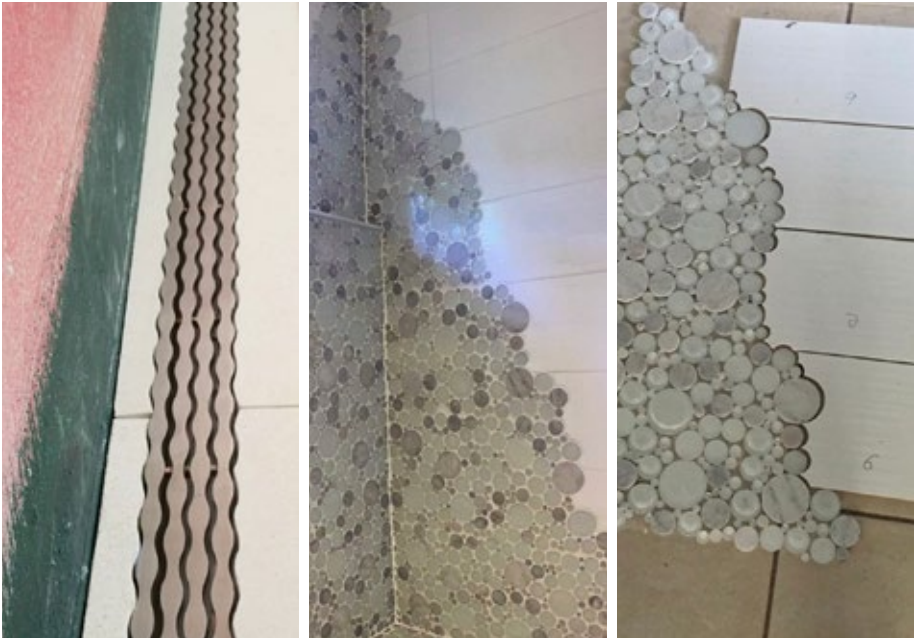
This was before scribing was cool and popular. The challenge for the bubble tile project was to precut all the field tiles (with lots of core bits and lots of time) to fit the bubble tile that was going in the corner. In the funky drain photo, Todd Neubauer hand scribed the field tile to fit the drain the homeowner bought.
